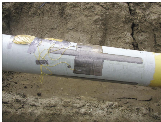
Bagging coils of sensor leads protects them from the weather before installation into conduit. One linear (parallel to pipe) and two coil sensors (either side of the linear) extend from the leads mounted on the pipe and are covered with a protective coating of epoxy (Fig. 8).
